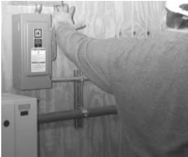
Figure 12-1. Proper method to safely bump or switch a disconnect lever on an electrical box.
