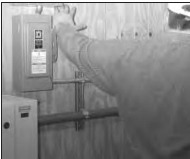
Figure 12-1. Proper method to safely bump or switch a disconnect lever on an electrical box.
