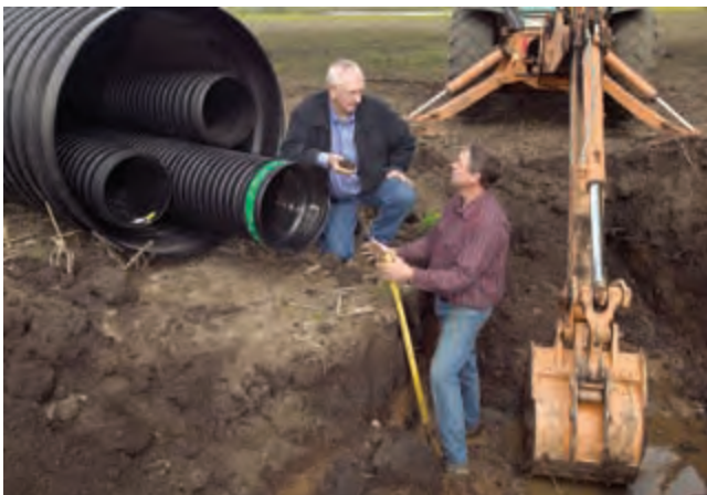
Figure 16. Installing a water control structure allows water levels to be manipulated and controls plant growth for attracting waterbirds and other wildlife. Photo by Peggy Greb, USDA Agriculture Research Service.
