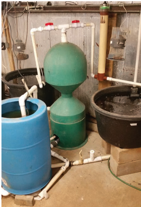
FIGURE 3. Two bead filters with slightly different shapes. Note the 2-inch top ports for water outflow, the 1½-inch drain ports at the bottom, the air-sucking side ports with the one-way check valve and the small 1-inch flash drain. The filter in the top photo uses a check valve on the exit port while the filter in the bottom photo uses manual valves. Backwashing this filter requires closing both valves.
