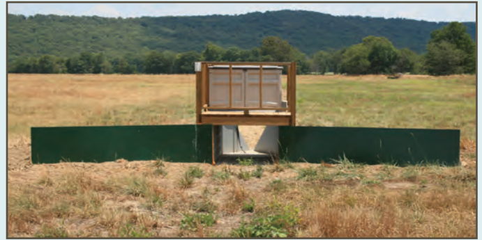
Water control structure for collecting runoff in pasture at Elkins.
