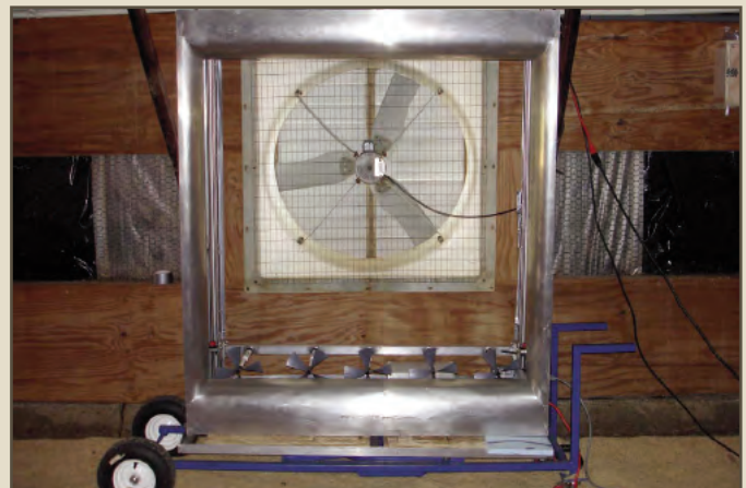
Top: Smoke tests are used to detect leakages in a poultry house.
