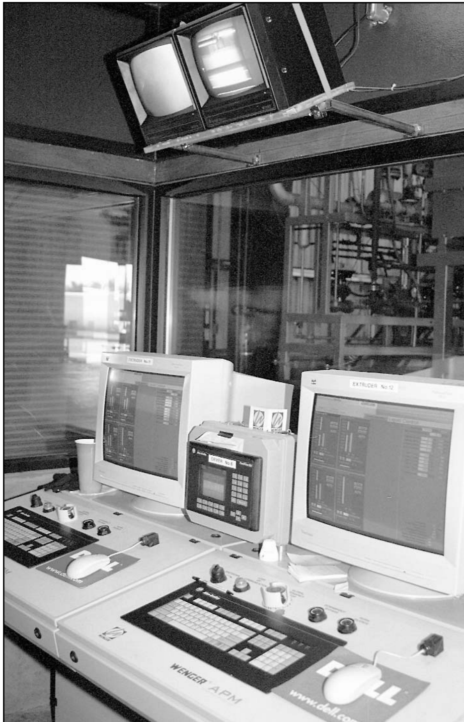
Figure 3. Control center for catfish feed mill.
