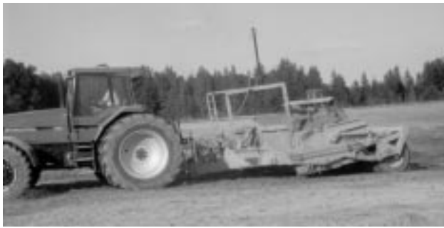
Operation of a laser controlled dirt pan on a field that is being precision graded.
